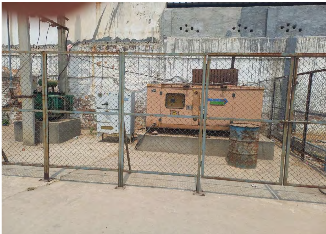
Fig: Generator to the capacity of 62.5 KWH installed in the college.
